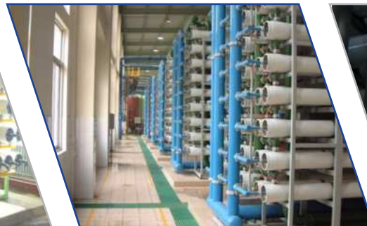
Biel Crystal water treatment engineering. May 2015
